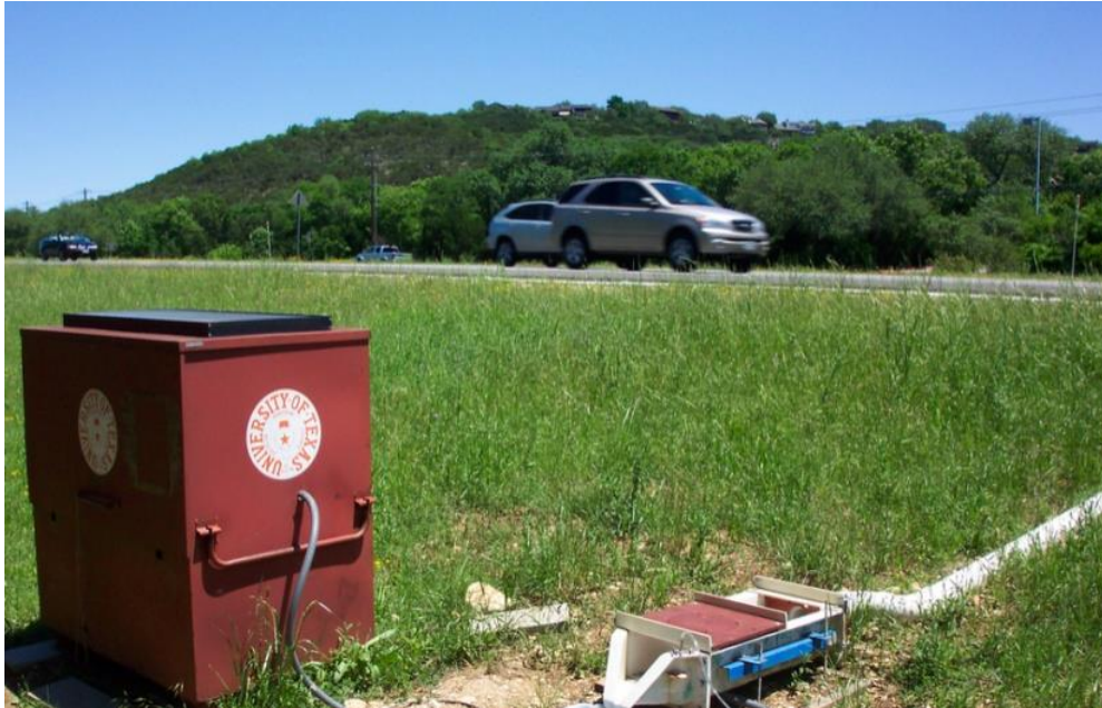
Figure 5. Photograph of H-flume and drainage pipe at Loop 360 monitoring site
